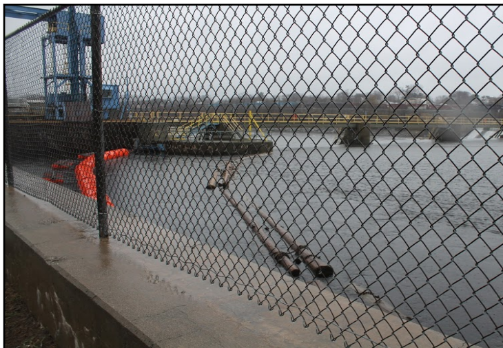
Existing boom positioned at dam intake on east side of river near location of EX-02.
